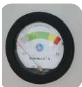
MANOMETER differential pressure gauge to monitor the filter life.
